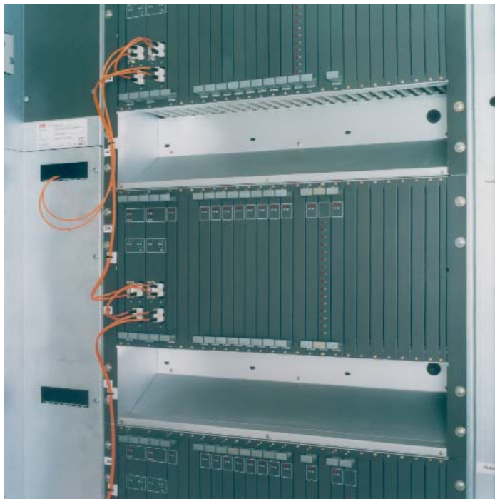
Racks within a station
